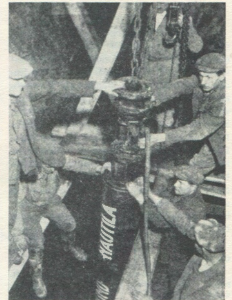
Figure 4. Installing one of the 'Nautilus' pumps in the Punkva Cave. Photo by Karel Absolon.
